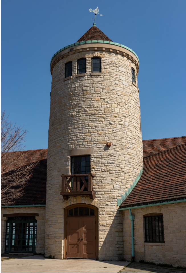
Left: The pavilion tower's rustic second-floor balconette has a balustrade of diagonal crosses. Directly below, the original paneled doors are still in place. Oak lintels are visible above the north wing door opening at left and the arched window at right. (Photo by Paul R. Burley via Wikimedia Commons)
